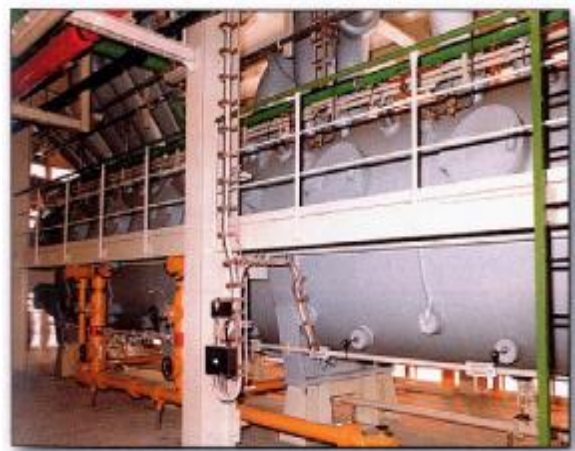
8-stage cooling crystallization plant/8 段结晶
