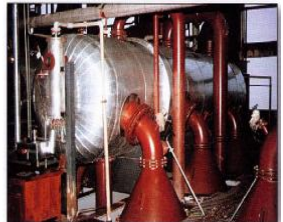
Evaporator and heaters/蒸发器和加热器
